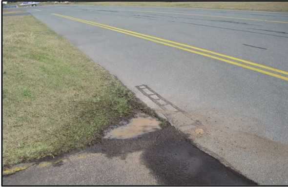
Figure 31 Example of leaving paved areas resulting in mud, grass and gravel on taxiway
