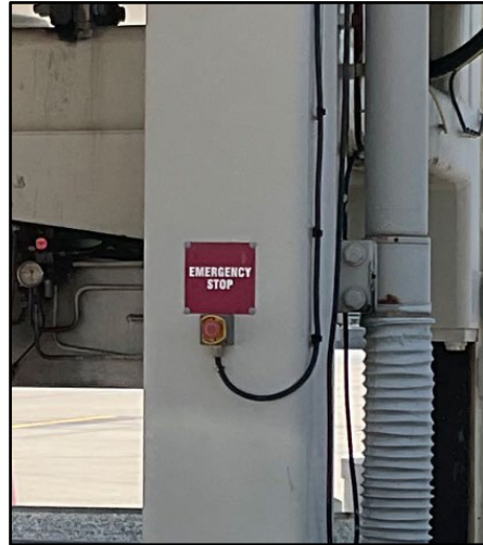
Figure 25 Aerobridge Emergency Stop Button
